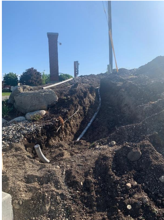
Figure 14: Conduit – Trailhead Golf Course
