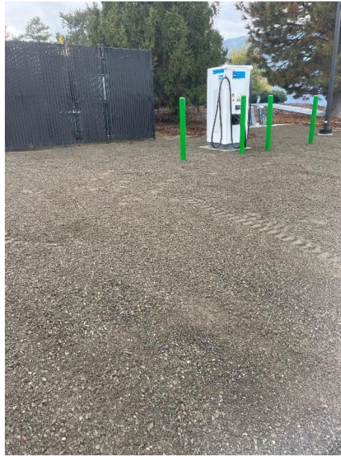
Figure 15: ABB Terra 184 DC Fast charger – Clarkston, WA DCFC Site
