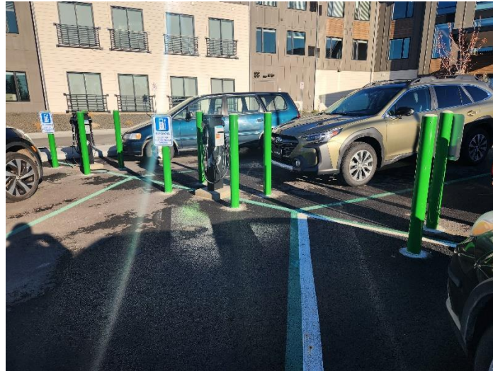
Figure 9: Multi-unit dwelling charging installation
