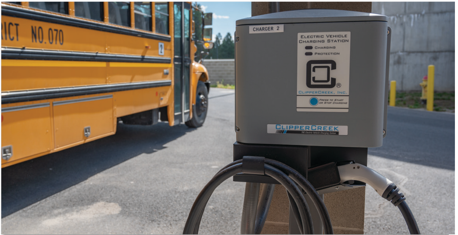
L2 electric bus charging at VL Transport in Valley, WA
