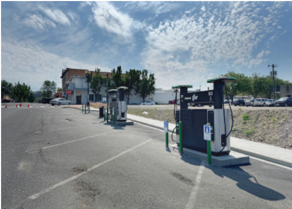
Flo Ultra 320kW DC fast charging stations in Colville, WA
