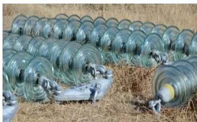
Strings of transmission insulators, sometimes called bells
